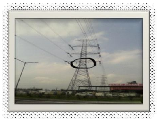
Fig 3: Deposition of Pollution on Insulators
